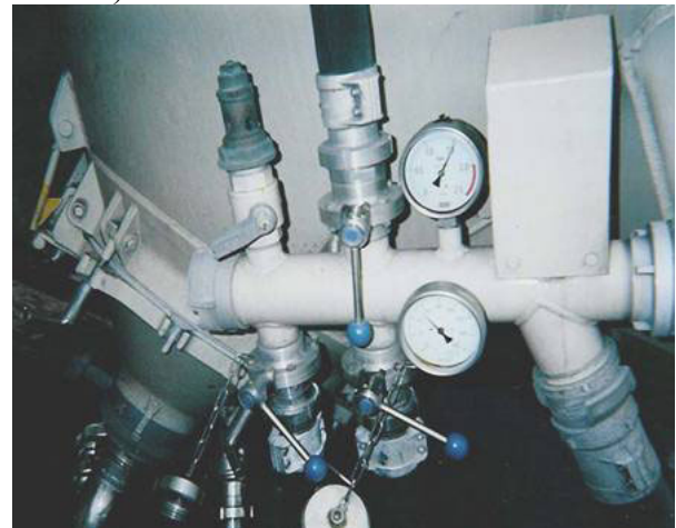
Air distribution valve during unloading.
